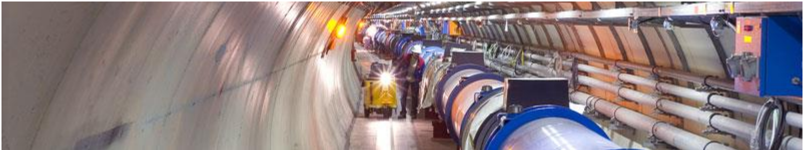
3000 RADFETs installed in the LHC ring at CERN
