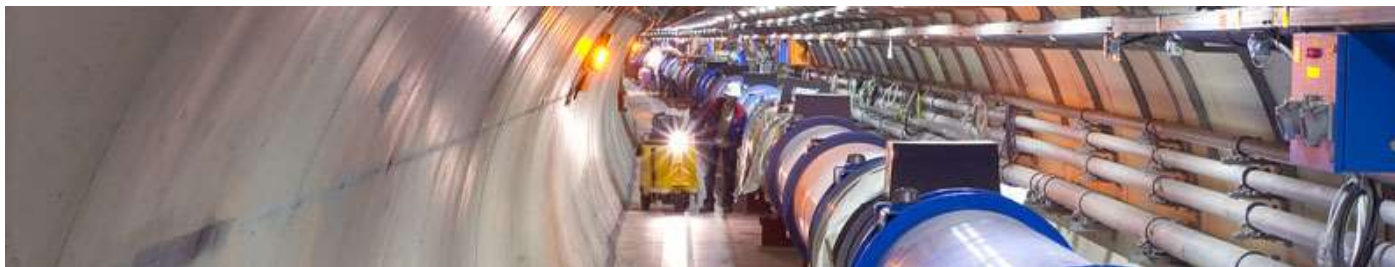
3000 RADFETs installed in the LHC ring at CERN
